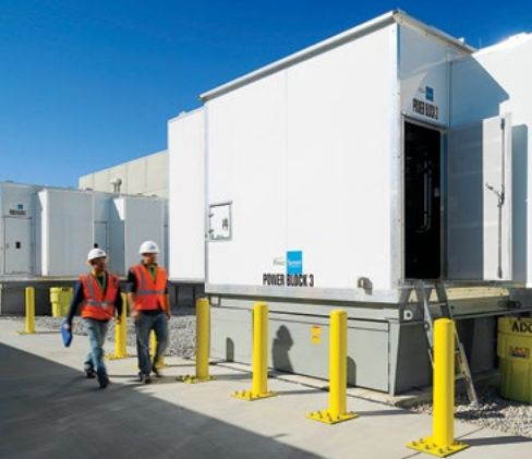
PowerSecure staff inspect a PowerBlock® generation unit in the equipment yard at Aligned Data Center's Plano, Texas facility.
